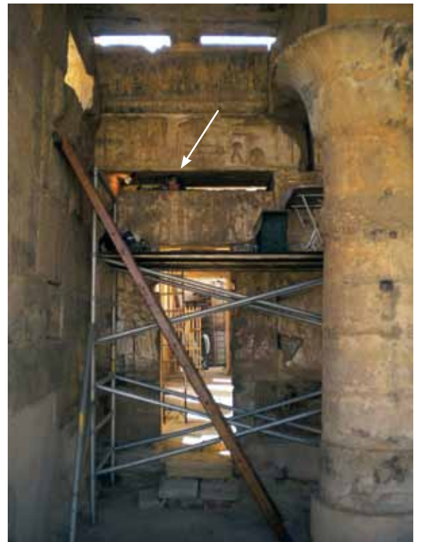
Sue Osgood inside the Akoris lintel at the top of the scaffolding at Medinet Habu
